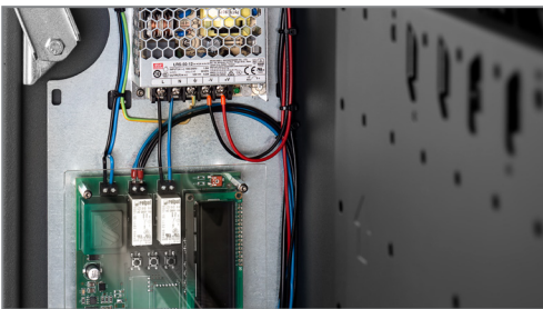
Cabling according to VDE guidelines
